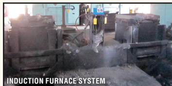
INDUCTION FURNACE SYSTEM
